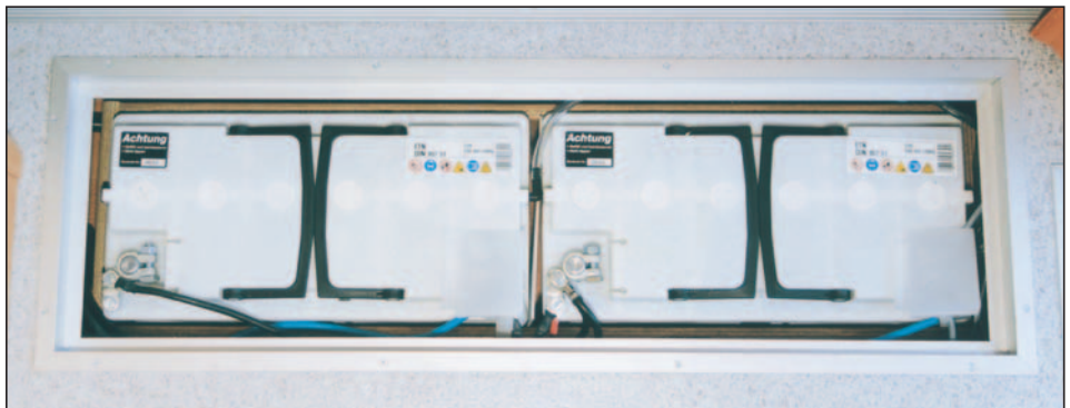
Current needs are well taken care of by two 105 amp hr leisure batteries accessed via a hatch in the floor. The 12V control panel has a digital display.
